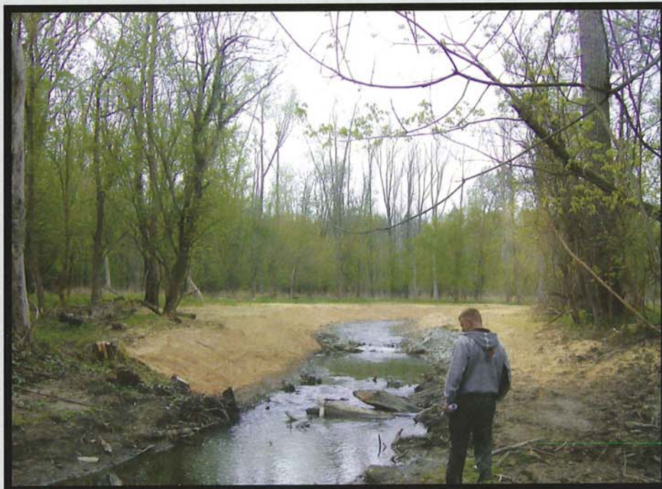
City of Elyria's Project Engineer, Aaron Klein, inspecting the end result of the Ridgeway Ditch Restoration Project.
